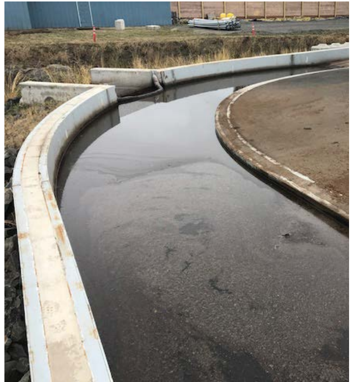
The concrete forebay allows sediment to settle out of site runoff into a concrete channel, where it is easily removed.
