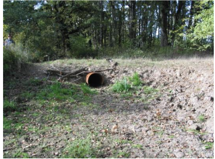
This undersized culvert blocks fish passage on the historic Coyote Creek channel bed.
