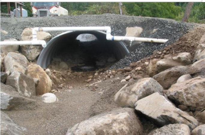
Post-project: The new 66" by 51" culvert was bedded with river rock to create a natural stream bottom.
