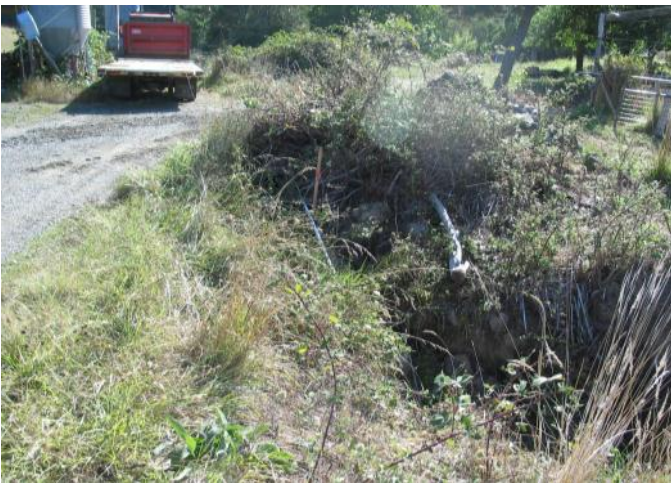
Pre-project: The 18" culvert was undersized and its outlet was perched above the stream.
