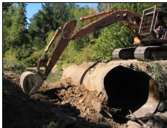
An excavator removes the undersized culvert that blocked fish passage to 46 miles of upstream habitat.
