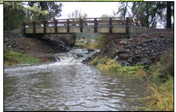
Before & After: The top photo shows the two foot drop at the culvert's outlet in the summer. Now the crossing is passable to fish year round .
