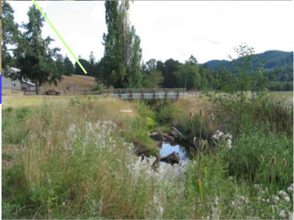
Post-project: We replaced the culvert with this bridge that provides year-round cutthroat trout passage and decreases downstream erosion.
