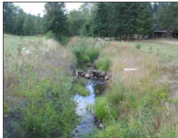
Post-project: Culvert was removed. Rock weirs were installed to prevent further stream incision. Blackberry was removed and willows, shrubs and trees were planted along stream banks.
