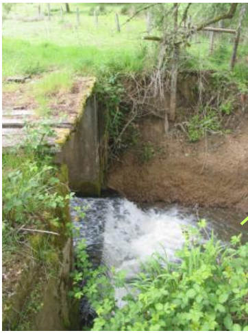
Pre-project: This irrigation dam, downstream of the culvert, also blocked fish passage
